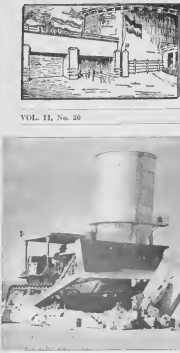
THE HOSPITAL WALL crumbles under pressure of a bulldozer. The wall is being removed in preparation for temporary parking and entrance facilities during construction of the new fireproof wing.
